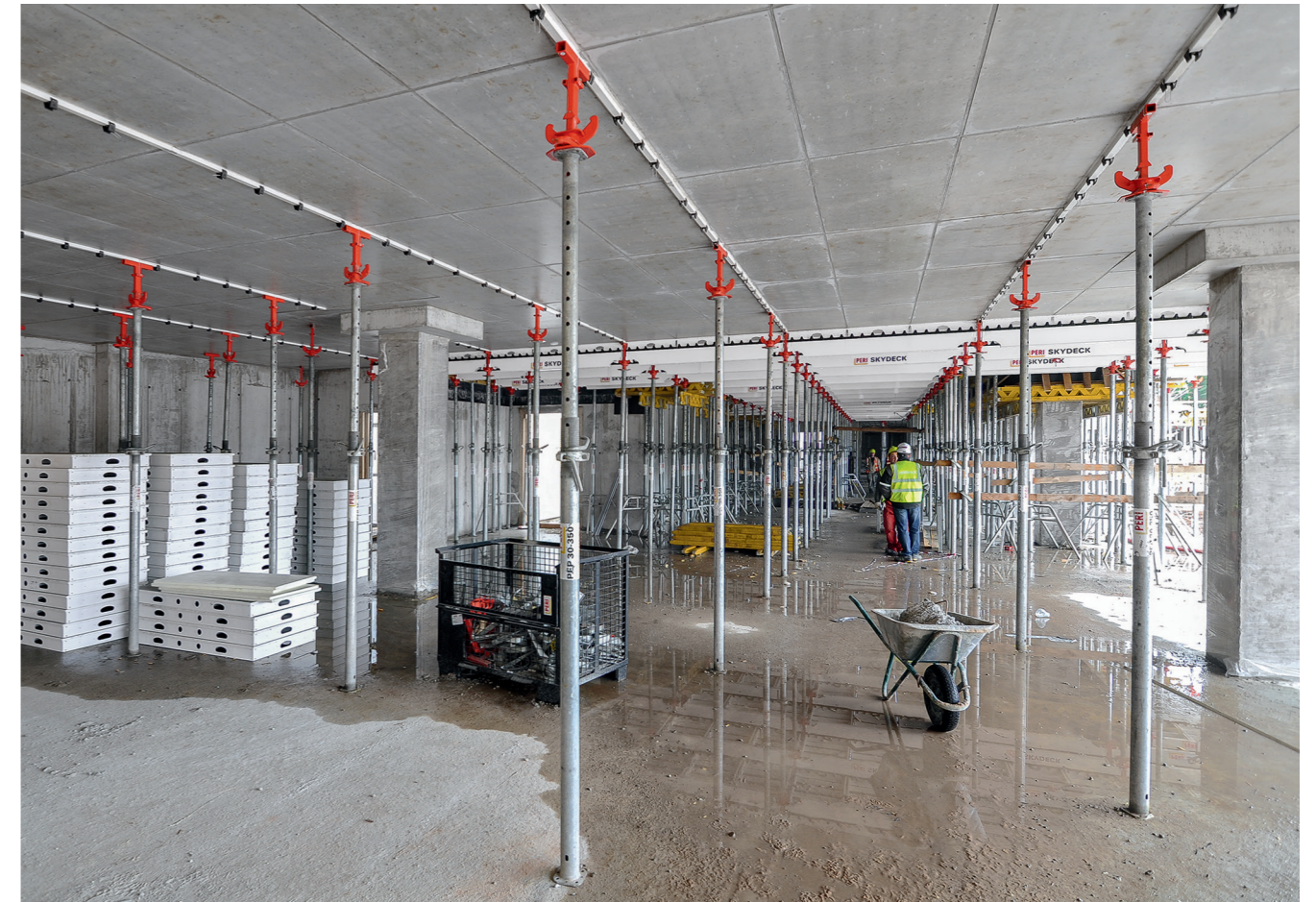
After early striking is finished, only the props with dropheads and cover strips remain in place. SKYDECK panels and beams are available for use in the next cycle.
