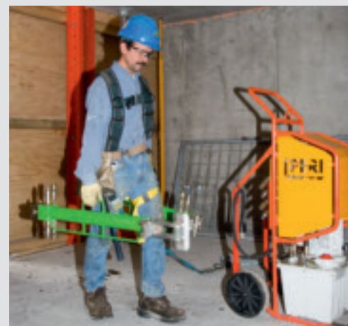
The hydraulic pump and cylinder are quickly operational.
