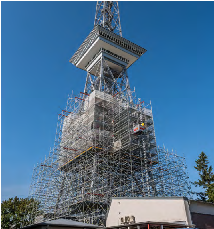
The old paintwork had to be removed and new corrosion prevention added, while the steel structure had to be completely re-painted.
