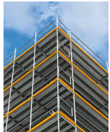
To form outside corners, you only need a frame column – all you then have to do is fit your decks on the horizontal ledger of the adjoining scaffolding bay.
